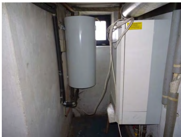
Kotel a boiler v 1.PP
